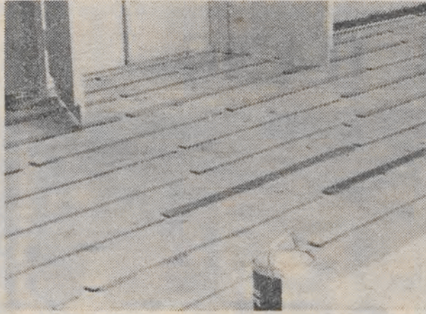
The floor of the Sports Hall. "The wood was found to be rotten."
