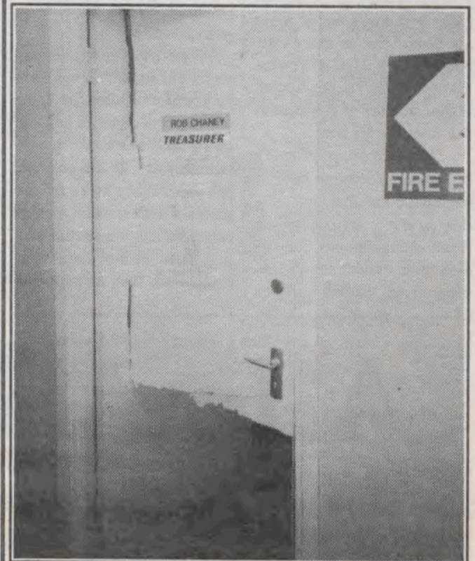
An example of the damage caused to the Mandela Building after the break-in.
